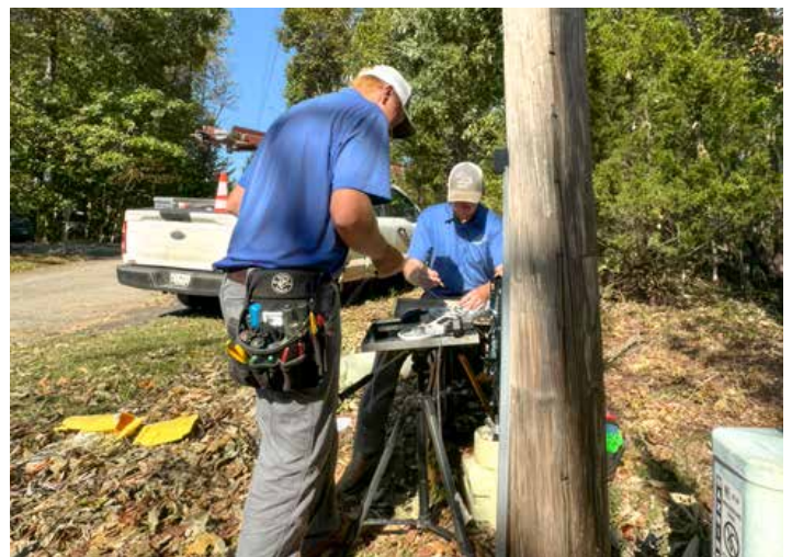
Construction technicians Mason Johnson, left, and Andrew Price work to repair West Carolina’s network after Hurricane Helene.
